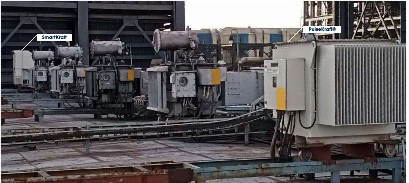
Figure 5: Power supply installation on field 1-6 out of 7 fields. SmartKraft is in field 1 and field 6 is equipped with PulseKraft®
