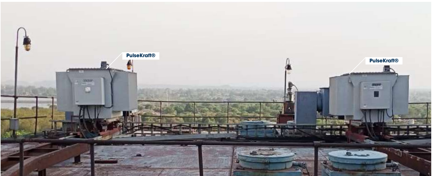
Figure 6: Field 6 and 7 are equipped with PulseKraft®
